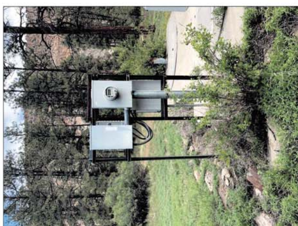
EXISTING CONTROL PANEL AND STATION SERVICE
