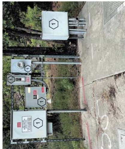
OVERALL CONTROL PANEL AND ELECTRIC GEAR
