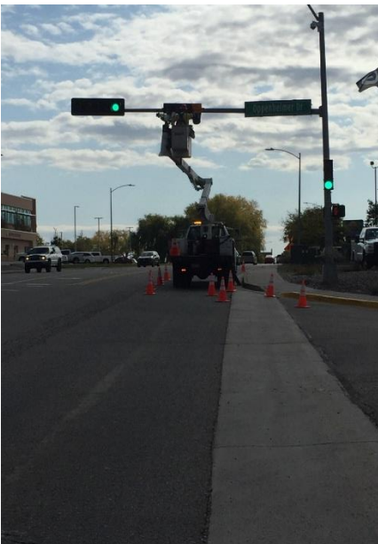
Traffic Electricians installed a 4 section signal head at Trinity Oppenheimer. This fixture replaces a 3 section signal head adding a 2nd red to help motorists with visibility issues associated with the fall sunshine during the morning commute.
