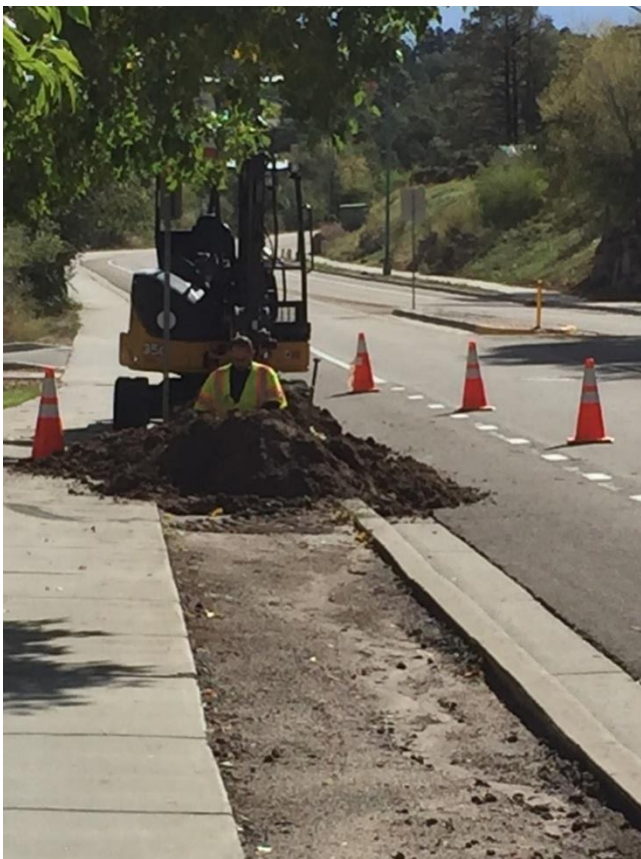
Traffic Electricians trenched along Canyon Drive to relocate a street light near a transit stop.
