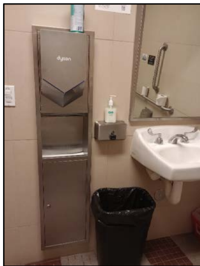
To reduce the usage of paper towels and to prevent future sewer clogging, Facilities construction specialists installed electric hand dryers in the shower rooms located at the Municipal building ground level by the employe entrance door.
