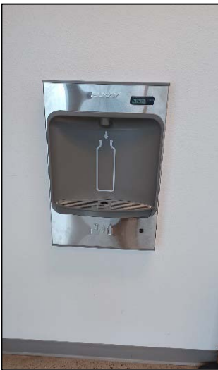
Bottle filler installed at NPS Visitor's Office
