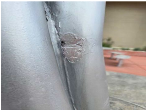
Detail: Area of failed paint pulled back to a stable point and then painted.
