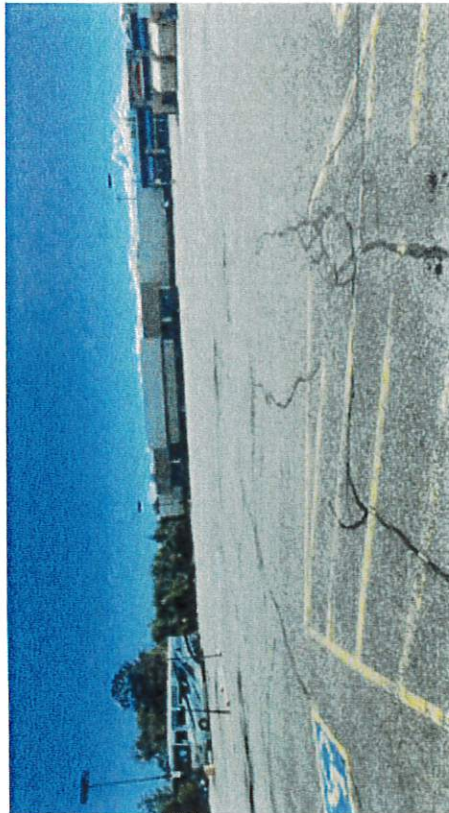
Figure 17. Deteriorating pavement on roadways and side streets is present throughout the proposed MRA
