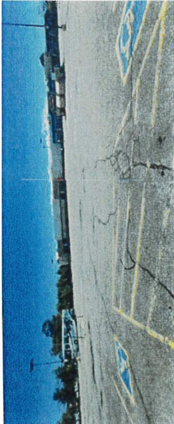
Figure 6. Extensive underutilized and deteriorating surface parking lots are present throughout the MRA
