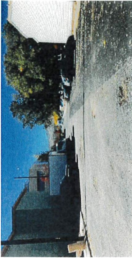
Figure 18. Deteriorating pavement on roadways and side streets is present throughout the proposed MRA
