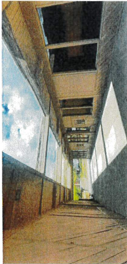
Figure 10. Entirely vacant building in the Mari Mac Shopping Center
