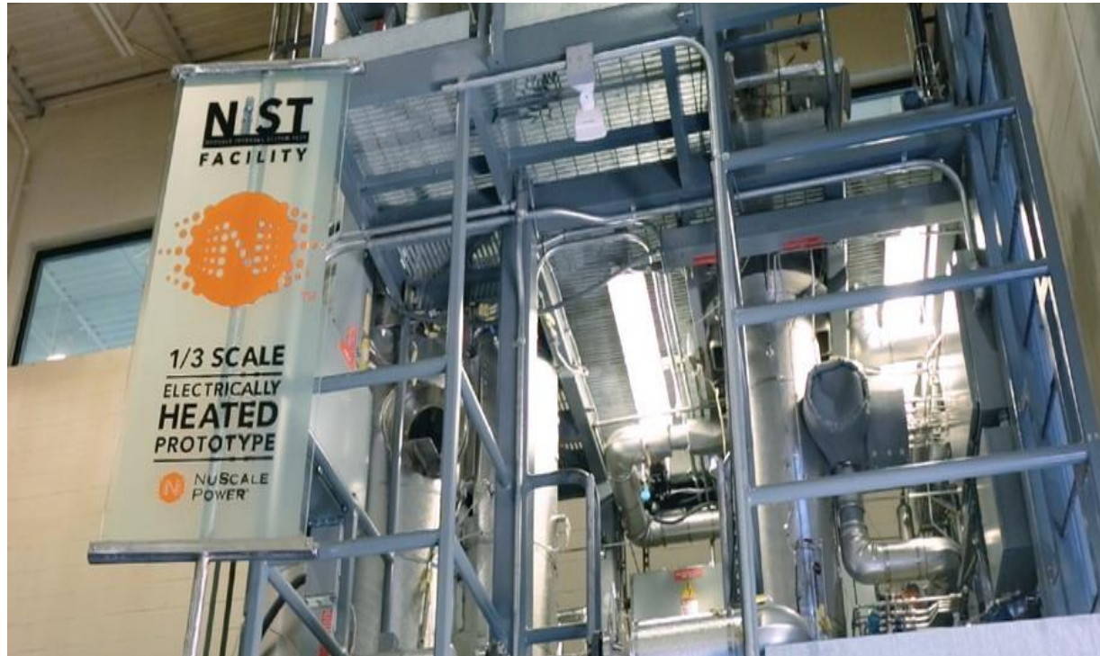
NuScale Integral System Test (NIST-1) facility located at Oregon State University in Corvallis, Oregon
