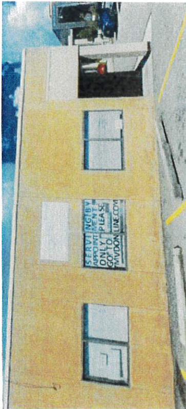
Figure 15. Deteriorating buildings are prevalent throughout the proposed MRA
