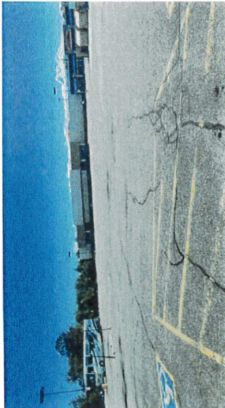
Figure 17. Deteriorating pavement on roadways and side streets is present throughout the proposed MRA
