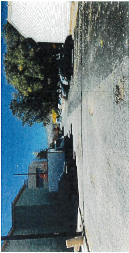
Figure 18. Deteriorating pavement on roadways and side streets is present throughout the proposed MRA
