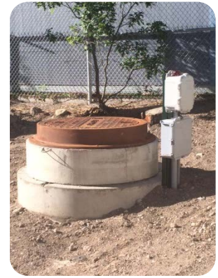
New Lift Station
