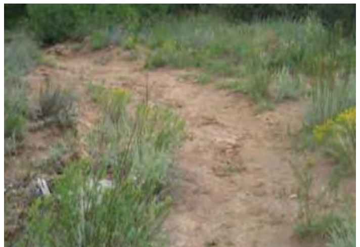
Monitor erosion at trailhead on Barranca Road.
