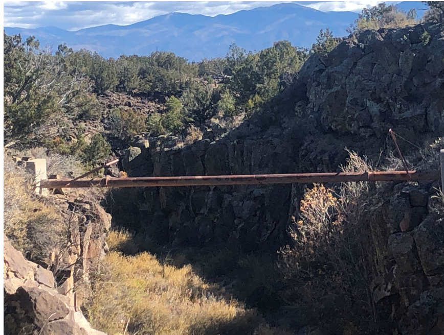
Figure 24: Pajarito Force Main Crossing Looking West
