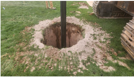
Netting Pole Hole
