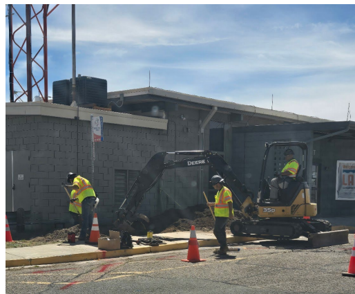
Facilities construction specialist members of the crew repairing a leak in the main line supplying water to the airport. This photo clearly shows the complexities and effort level in the work conducted by Facilities to provide immediate response to emergencies around the County.
