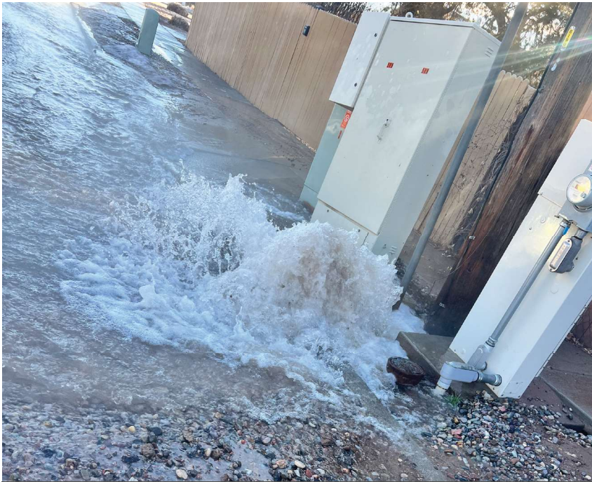
GWS crews responded to a water break on Rover Blvd. in White Rock and replaced about 8 feet of pipe due to a 4-to-5 foot crack ran along a 10" cast iron main.
