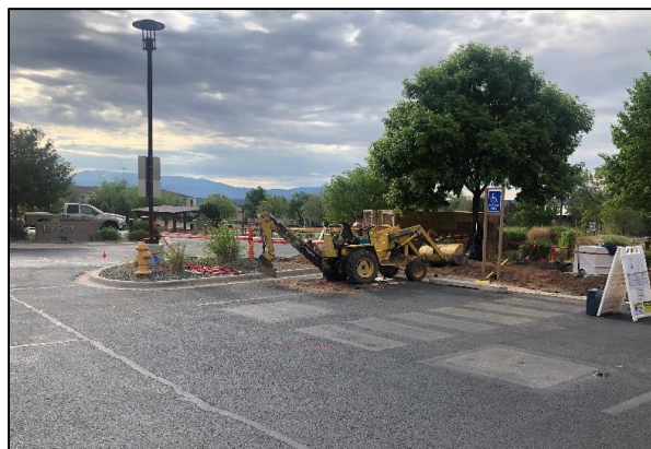
Construction is underway at White Rock Visitor Center to improve water pressure to the building. Trenches are being hand-dug to avoid striking underground utilities.
