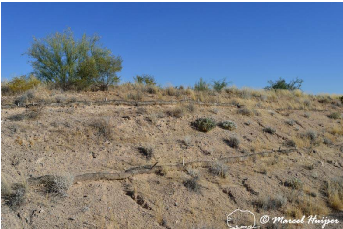
Figure 56. Straw fiber rolls to control erosion on a road cut, Hwy 87, Arizona, USA.
