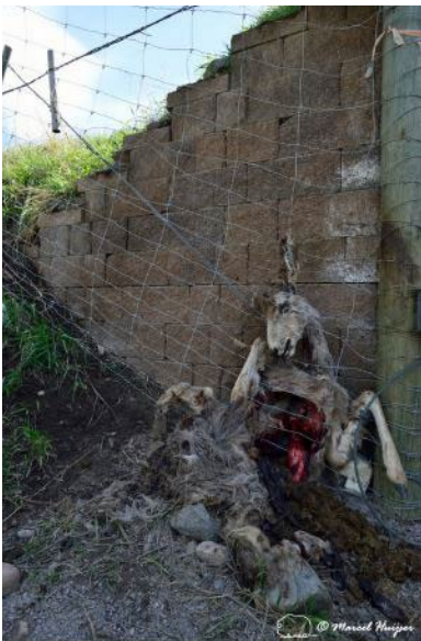
Figure 53. Mule deer ( Odocoileus hemionus ) got stuck between wildlife fence and the wing wall associated with a wildlife underpass and dies, Montana, USA. The fence should be snug up to the wing wall. Here the last fence post was close enough to the wing wall but the second to last post allowed for a funnel like configuration making the deer believe it could potentially pass in between the wall and the fence. When it realized it could not go forward anymore it tried to turn itself around and then got stuck and died. It is important that both the post and the fence are positioned such that no space is left between the wing wall and the fence.
