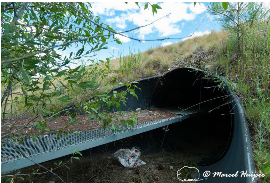
Figure 93. Shelf for small mammals in culvert originally designed for hydrology only, US Hwy 93 South, Montana, USA.
