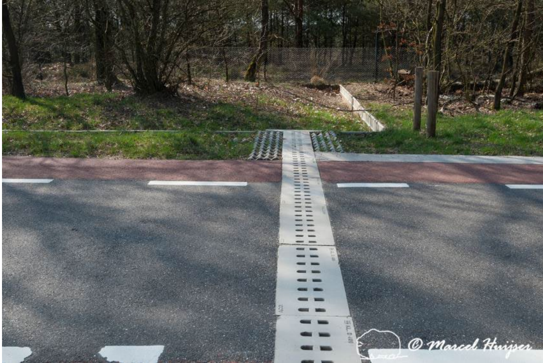
Figure 96. Amphibian tunnel with open slotted roof and barrier or wall for amphibians, integrated into roadbed, Deelenseweg, between Hoenderloo and Arnhem, Gelderland, The Netherlands.
