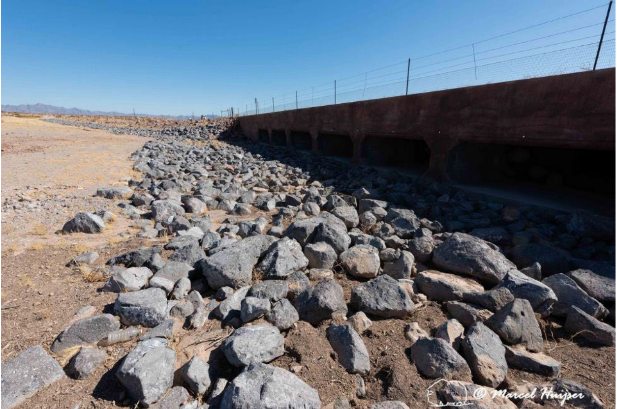
Figure 108. Riprap in front of culverts to reduce erosion, but the boulder are a barrier to Mojave desert tortoise ( Gopherus agassizii ), I-11, near Boulder City, Nevada, USA.
