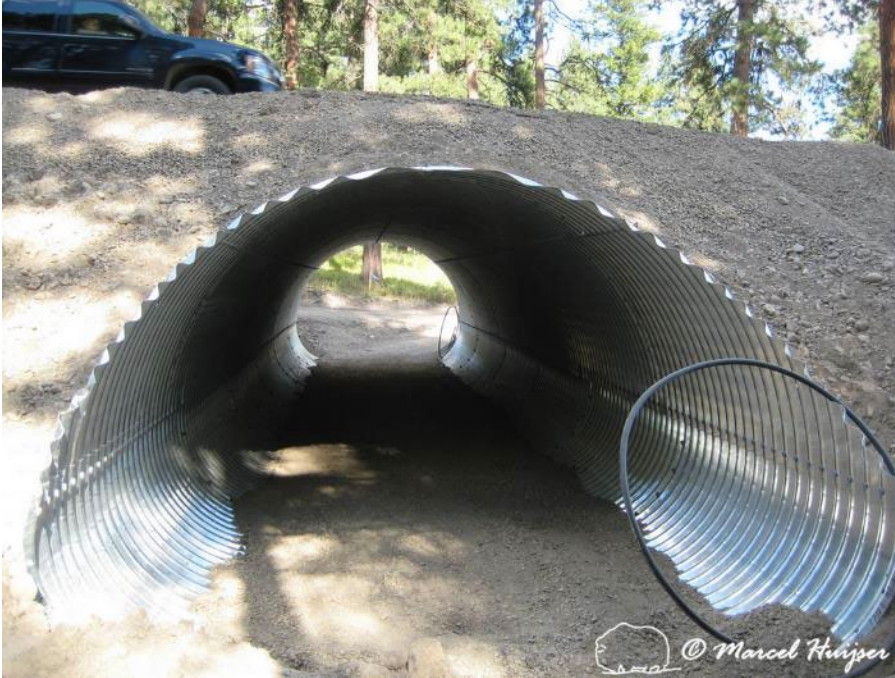
Figure 80. Corrugated metal culvert with soil covering the bottom.
