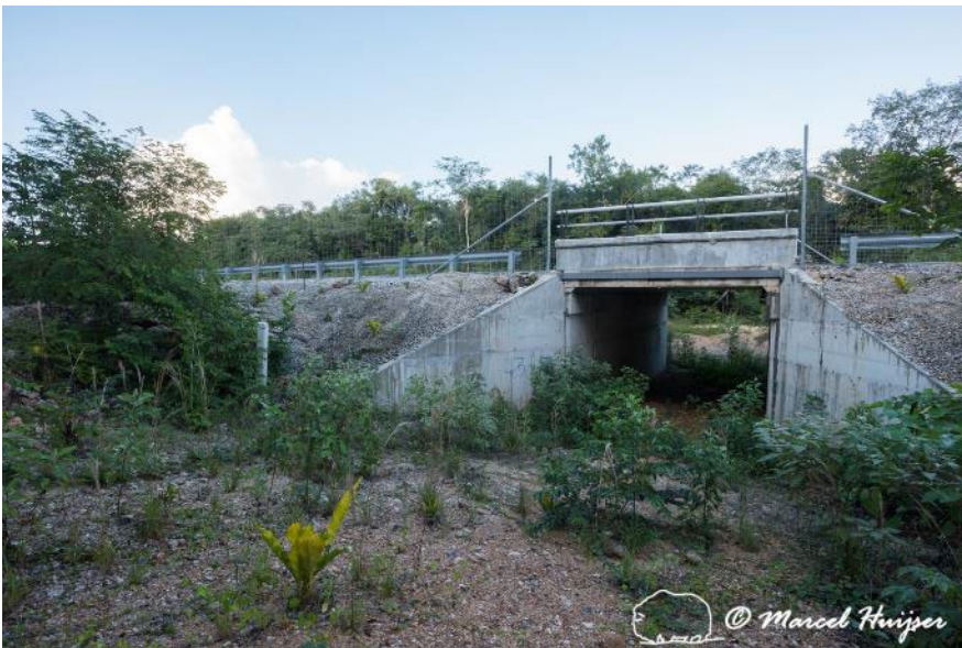
Figure 84. Wildlife underpass, Nuevo Xcan-Playa Del Carmen highway, Quintana Roo, Mexico.
