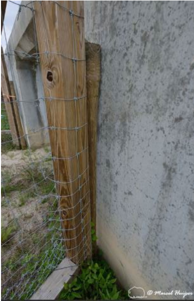
Figure 52. Tight connection (no gap) between last fence post and wall of the wildlife underpass, Hwy 331, Hwy 83 near Freeport, Florida, USA. The angle at which the fence comes in does not result in a dangerous wedge or funnel that could lead to animals getting trapped.
