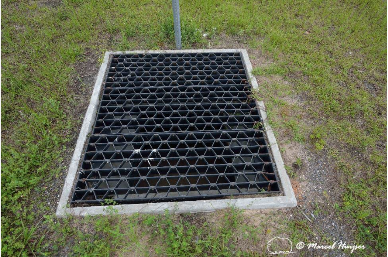
Figure 97. Opening (with bridge grate cover) in median to allow light and moisture in the wildlife underpass Hwy 331 Hwy 83 near Freeport Florida USA.
