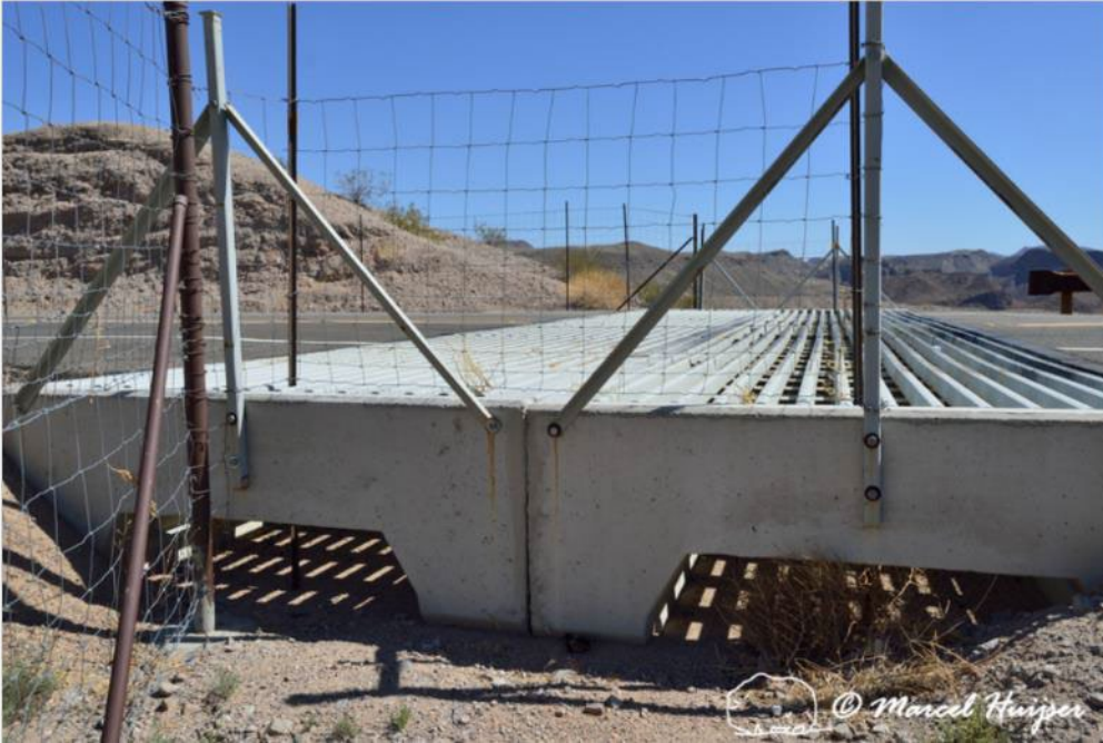
Figure 36. Combined drainage and escape for small animals under wildlife guard, Arizona, USA. The openings on the side allow for drainage under the culvert. The openings also allow invertebrates, amphibians, reptiles, small mammals and other species that may fall in between the metal bars to escape.
