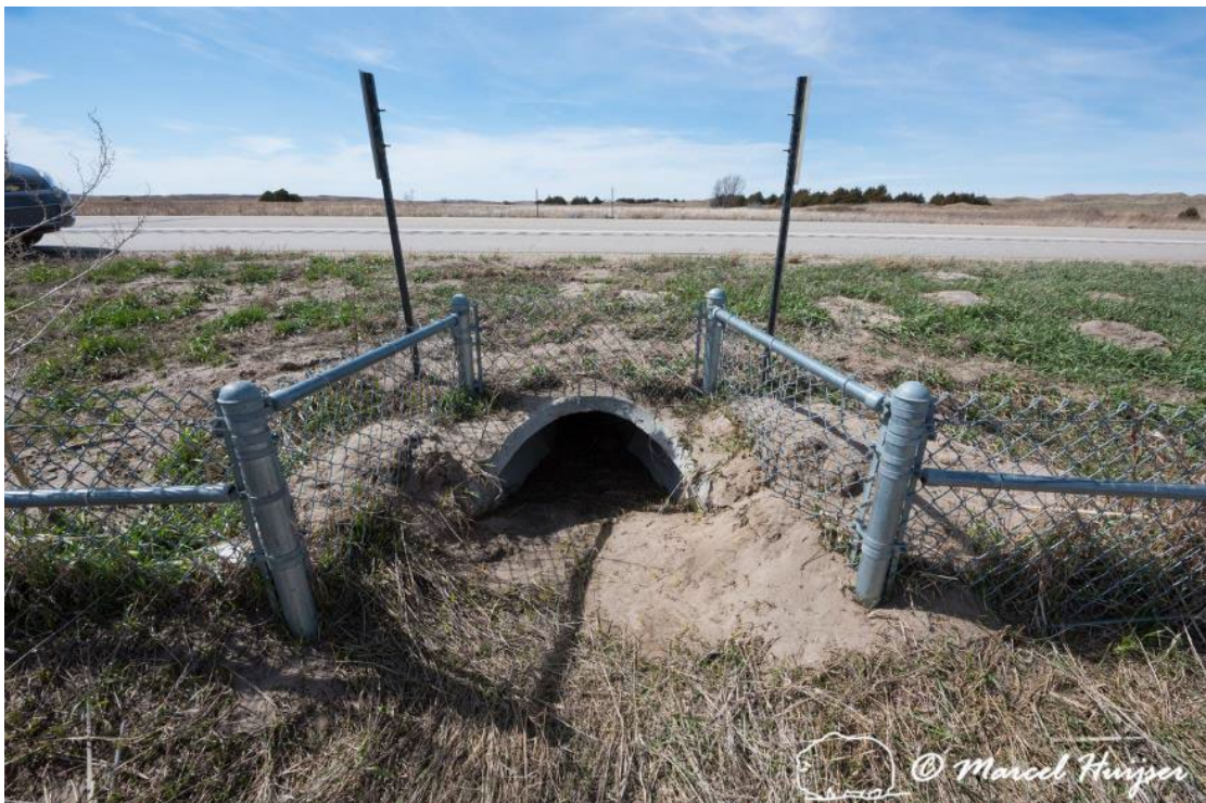
Figure 64. A chain-link turtle fence continues above a culvert for turtles, Valentine National Wildlife Refuge, Nebraska, USA.
