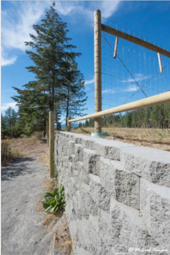
Figure 45. Wildlife jump-out with concrete blocks and a bar for bighorn sheep ( Ovis canadensis ), near Thompson Falls, Montana, USA. Note that it is probably better to not have the concrete blocks protrude as it makes it easier for species to climb the face.
