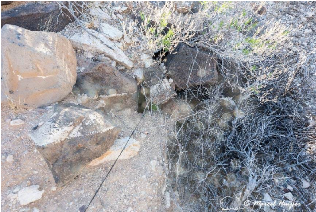
Figure 111. A culvert blocked by rocks under the road to the overlook, Childs Mountain, Cabeza Prieta National Wildlife Refuge, Arizona, USA.
