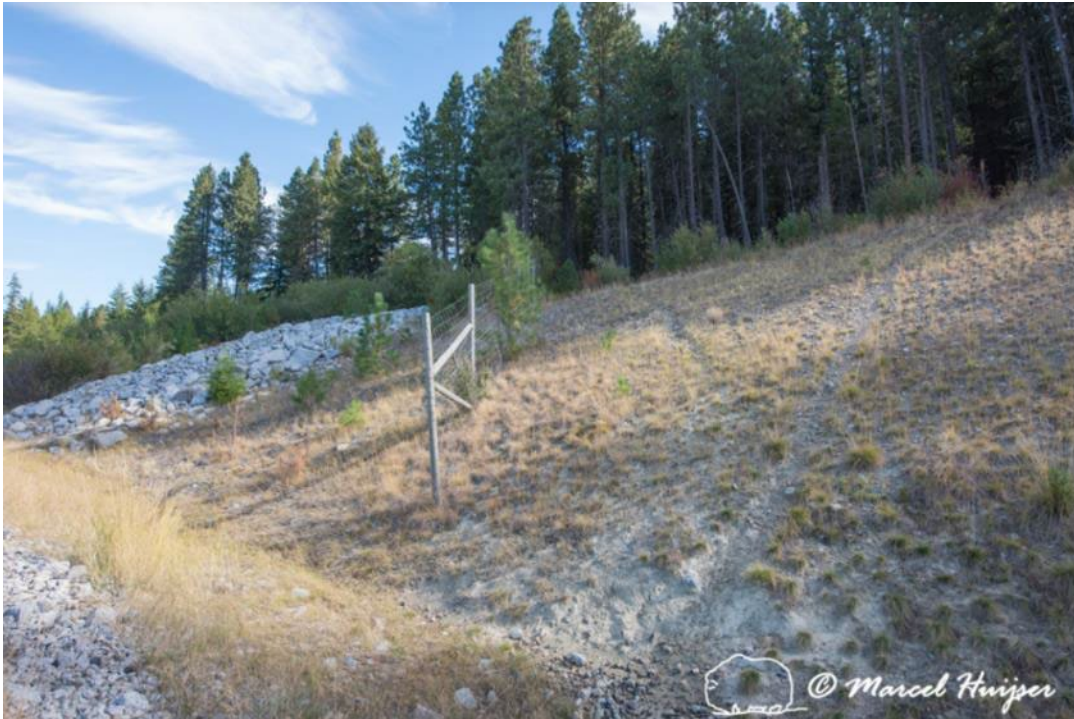
Figure 26. Wildlife trail at a fence-end, US Hwy 95, Bonners Ferry, Idaho, USA. This is an indication that there is a concentration of wildlife crossings at the fence-end (a "fence-end run"), potentially resulting in a concentration of collisions at or near the fence-end, just inside or just outside the fenced road section.
