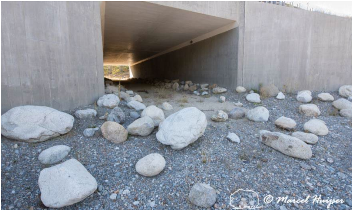
Figure 21. Boulders block access to unauthorized vehicles at wildlife underpass, US Hwy 95, Chilco, Idaho, USA.
