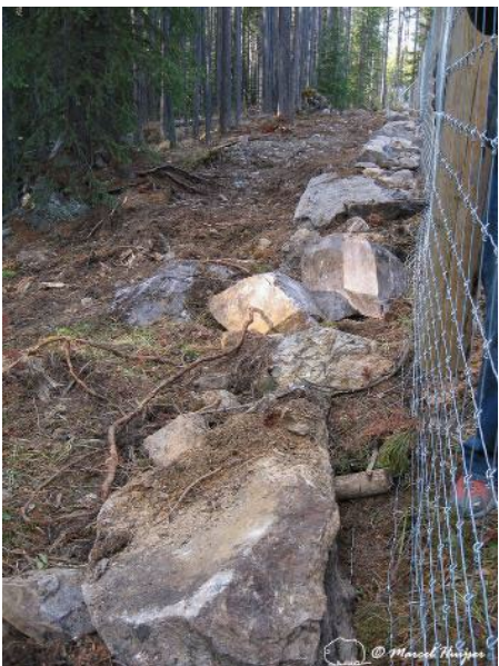
Figure 71. If a dig barrier cannot be dug into the soil, angling it away from the road and covering it with soil and rocks and boulders may be an option. Trans-Canada Highway, Banff National Park, Alberta, Canada.
