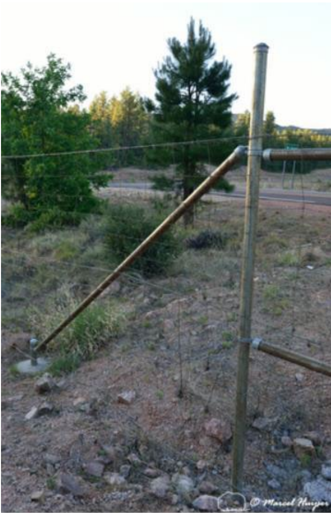
Figure 13. Wildlife fence with metal posts as a barrier for deer ( Odocoileus spp.) and elk ( Cervus canadensis ) along SR 260, east of Payson, Arizona, USA. Some of the metal posts are set in concrete.
