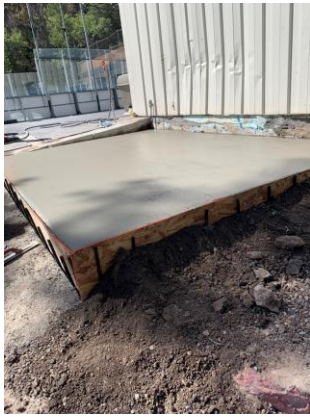
Slab of Concrete Parks Staff Made for New Shed at Ice Rink
