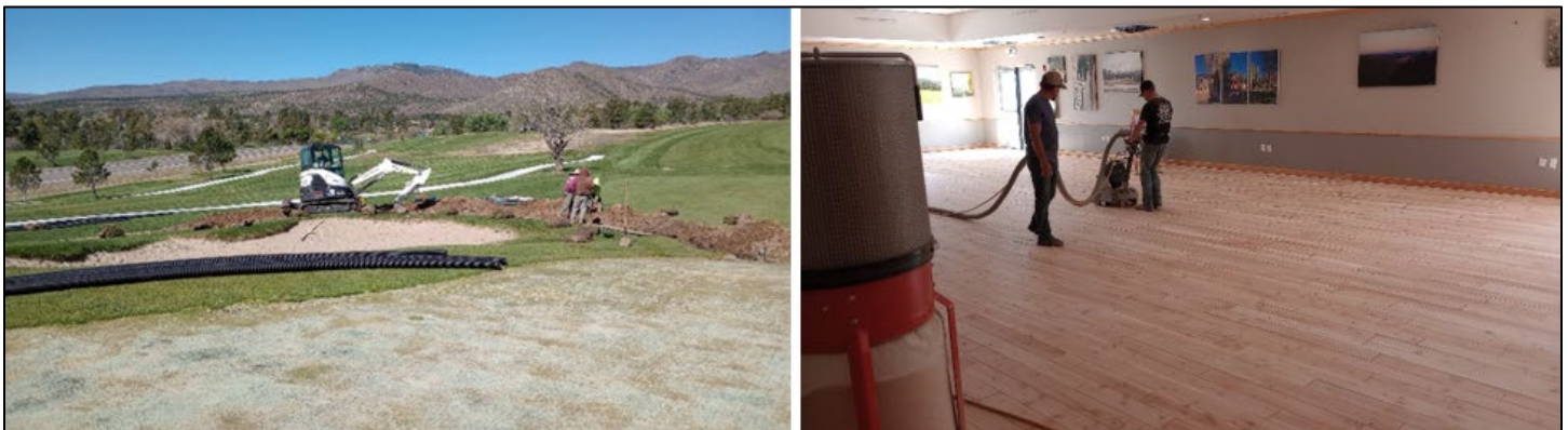
Drainage correction at Golf Course tees and greens. Contractors re-finishing the Community Room wood floors at the Golf Course Clubhouse.
