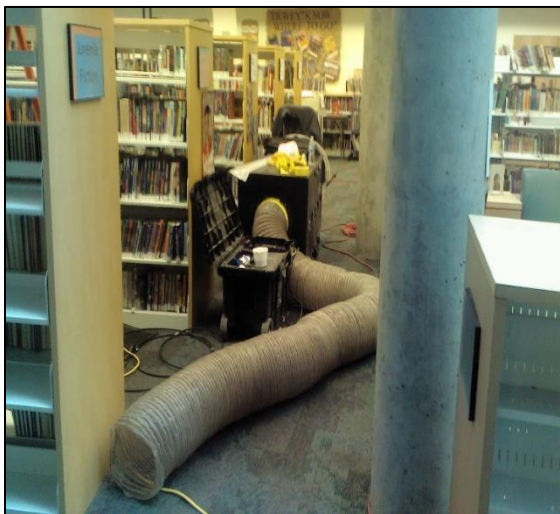
Youth area – duct cleaning equipment
