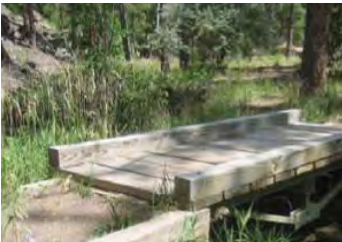
Monitor bridge condition.
