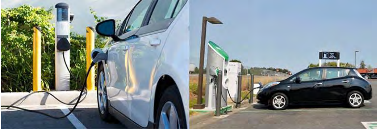
Figure 2-3: Level 2 charging examples
