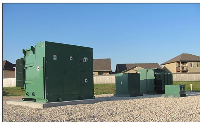
Figure -3: Modular Substation Example from Manitoba Hydro
