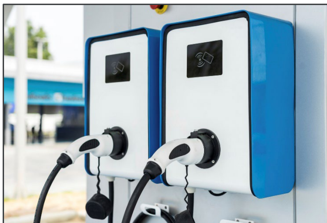
Figure -4: Electric Vehicle Supply Equipment
