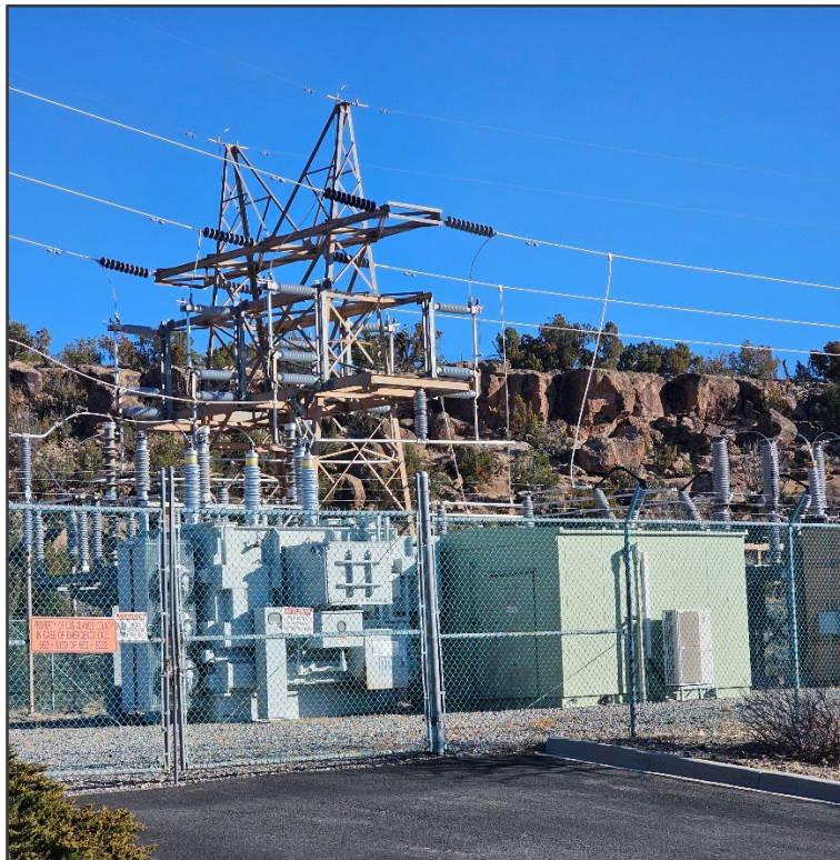
Figure -2: White Rock Substation
