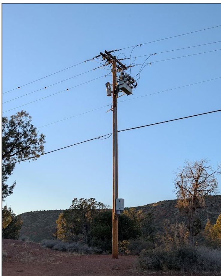
Figure -1: Distribution Line Recloser
