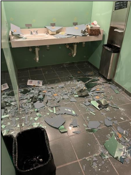
Facilities crews cleaned up a mirror that fell from the walls at the Betty Ehart Senior Center. Crews secured the remaining mirrors to prevent further mirror falling incidents.
