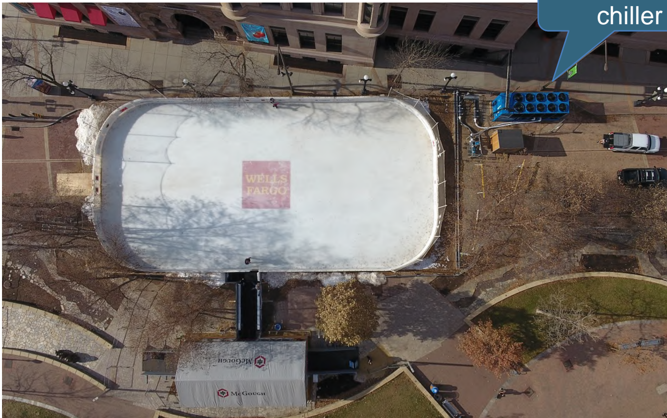
Temporary ice rink and chiller at Landmark Center in Downtown St. Paul, MN.
