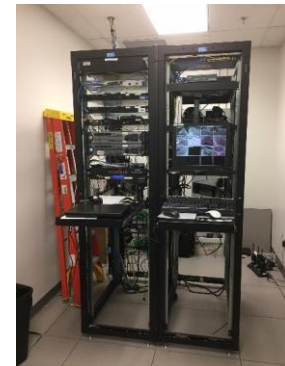
TMC Server Equipment
