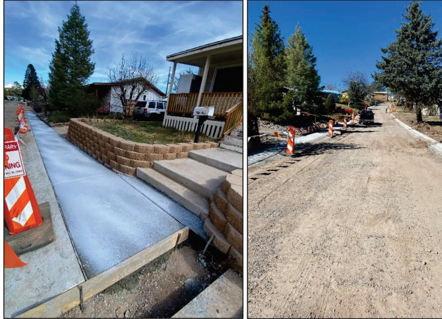
The joint project with the Department of Public Utilities includes full road reconstruction along with utility upgrades.
