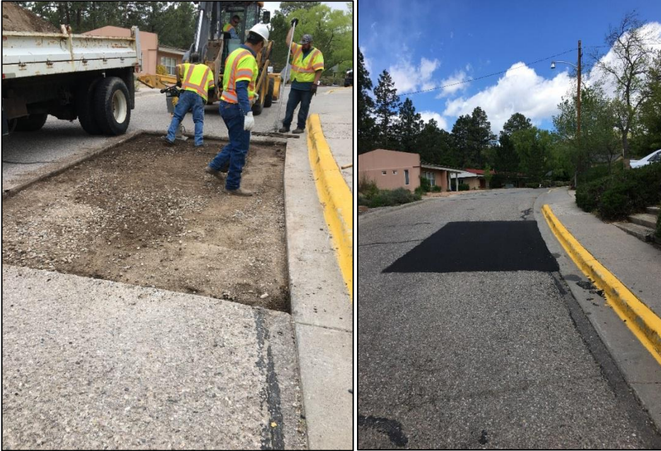
Crews are seen repairing a section of road on Fairway Dr. where utilities made a cut to repair a line.
