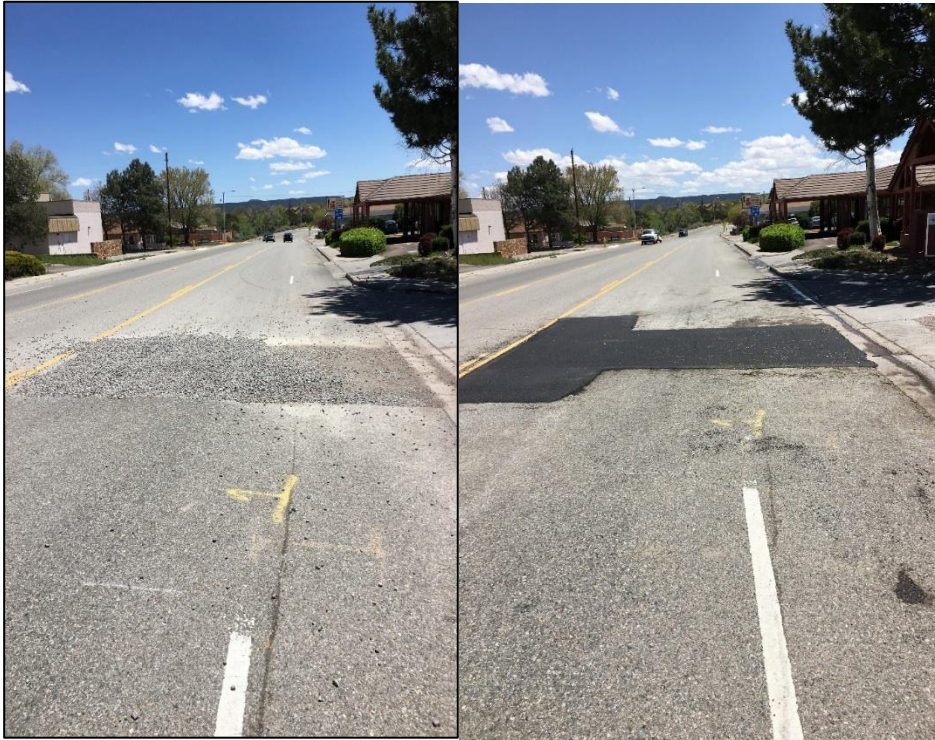
Crews assisted Utilities with an asphalt patch on Rover Blvd. where they had to repair a sewer main earlier this year.
