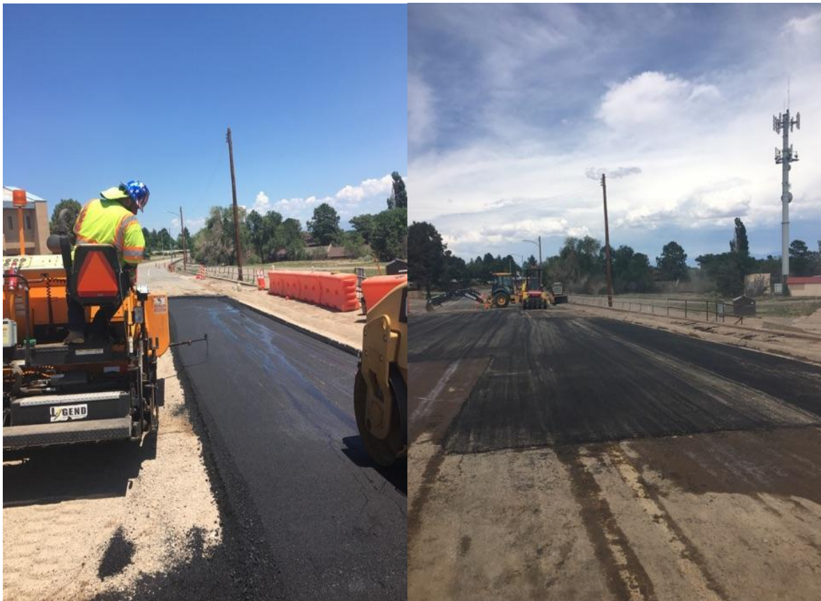
Crew members assist Utilities GWS on Trinity Drive between DP Road and 4 th Street where a sinkhole formed due to a leaking sewer main.
