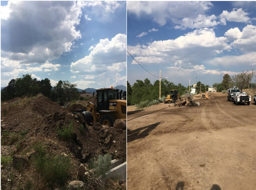
Crew members are seen clearing debris from vacant County land on DP Road.
