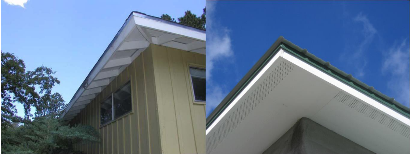
Rather than exposed eaves, the current interface code requires new construction to include eave protection from firebrands.
