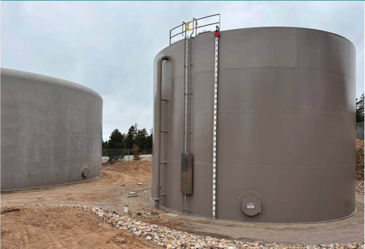
The new water tank constructed as part of the Jemez Mountain Fire Protection Project was completed during the third quarter.
