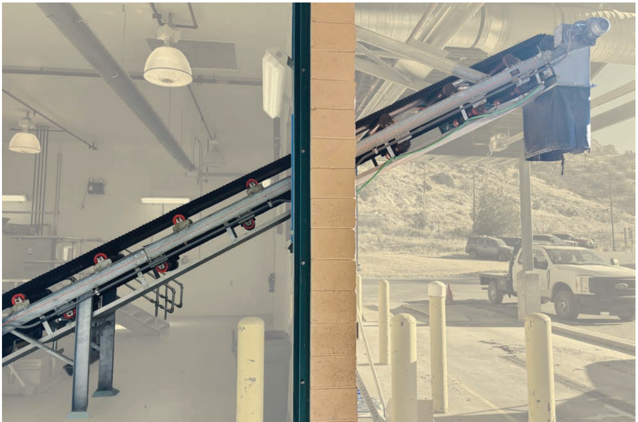
The new belt press at the Los Alamos WWTP is operational after a large replacement project.
