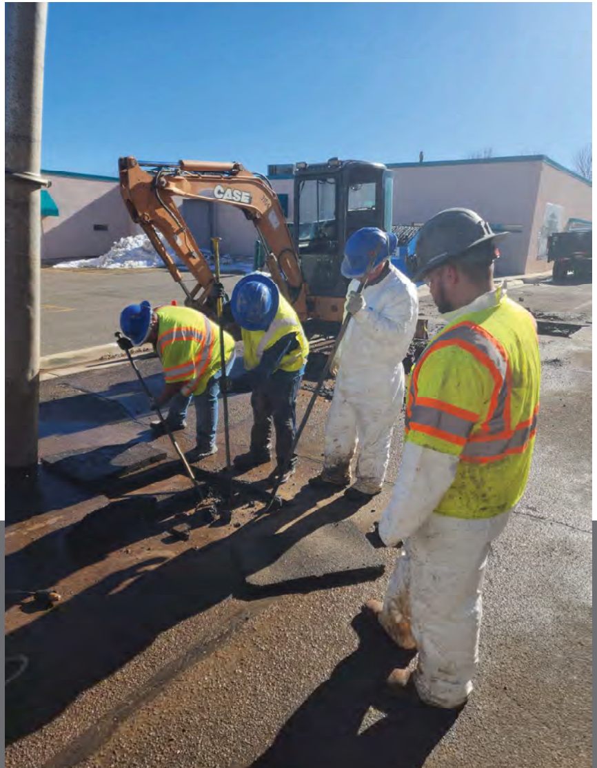
GWS crews repaired a broken water pipe behind Central Park Square in January.
