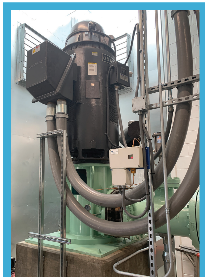
Construction of Otowi Well #2 was completed in FY2023. The total depth of the well is 2,310 feet, pumping from an elevation of 6,430 feet. The pumped water has a temperature of 84.4 degrees Fahrenheit.
