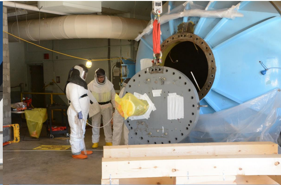
Horizontal Accelerator Tank Characterization
