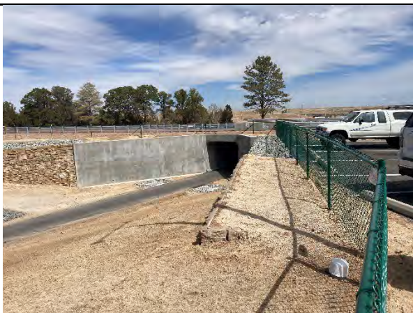
Below-grade connection across East Rd (502)
