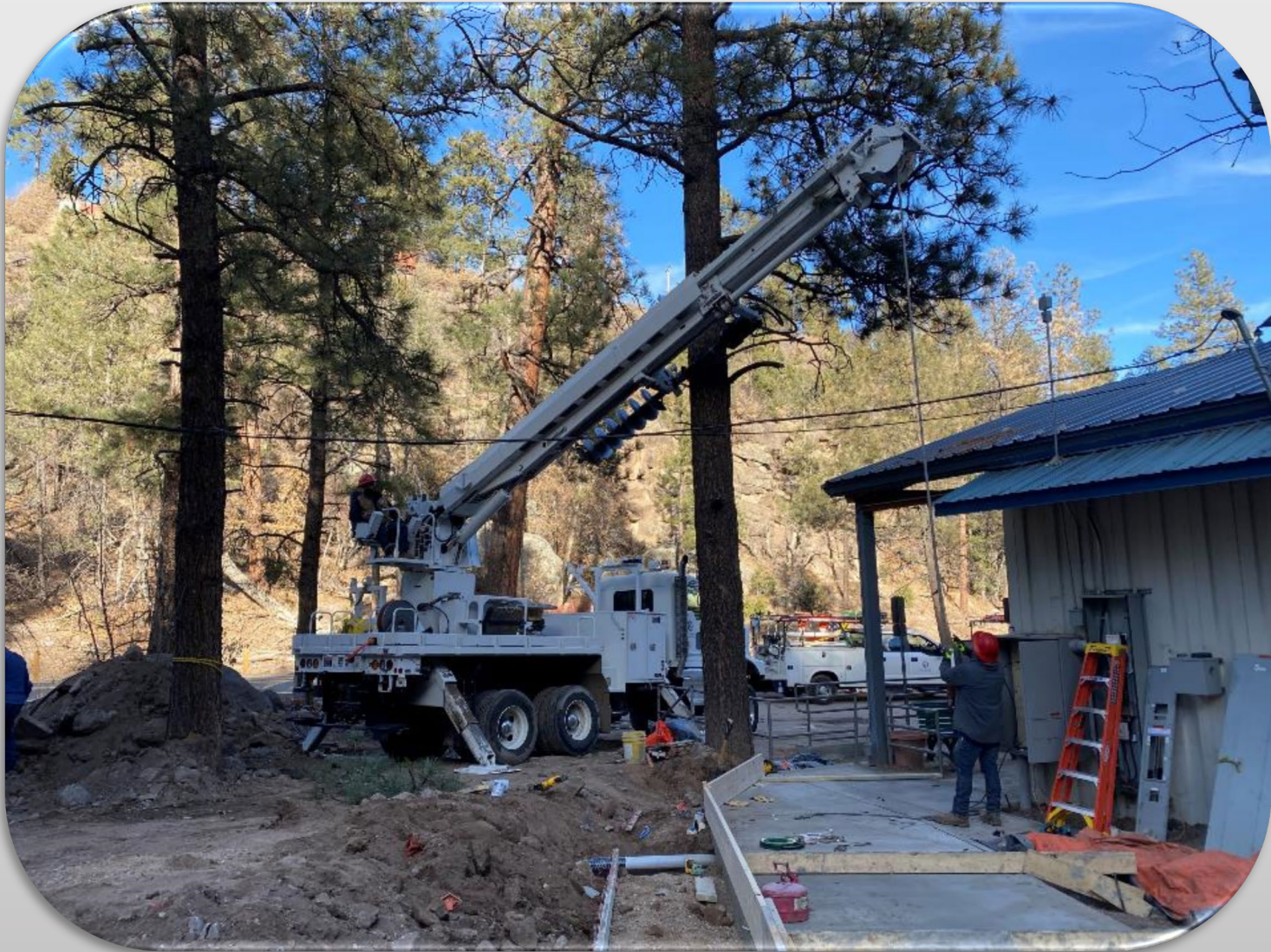
Contractor damage to primary service line at the ice rink
