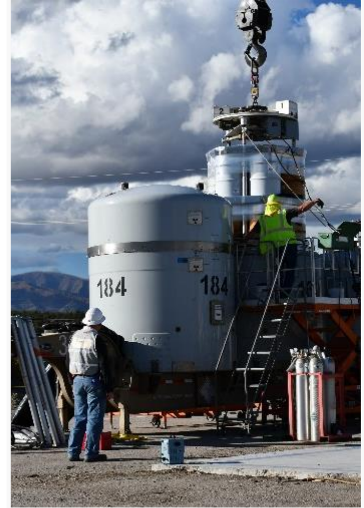
TRU Waste Mobile Loading
