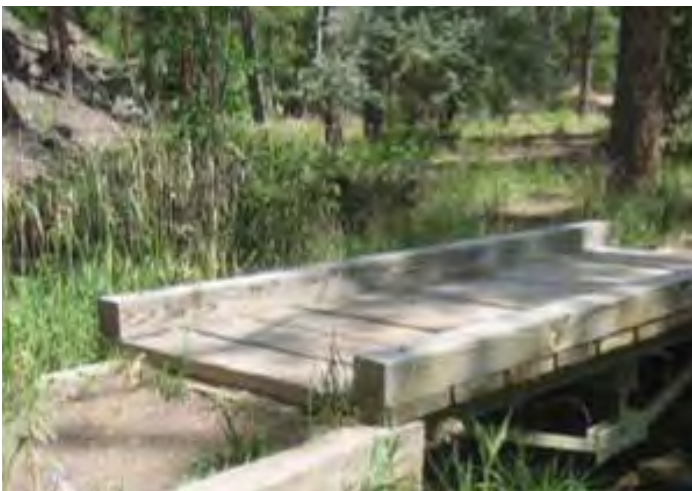
Monitor bridge condition.
