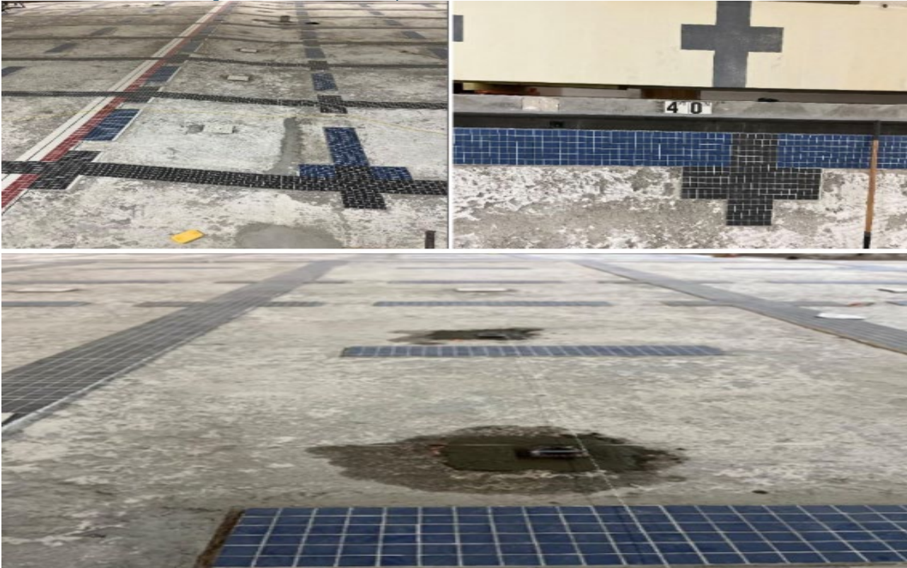
New Tile Installation Along Swim Lanes and Depth Indicators as Well as New Under Water Anchor Installed.
