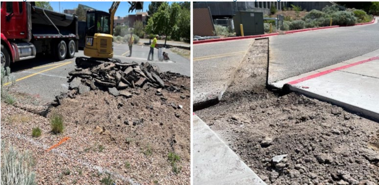
Mesa Public Library EV charging station project: crews trench and remove asphalt to run new electrical conduit from the existing transformer to the future transformer location in the reconfigured parking area.
