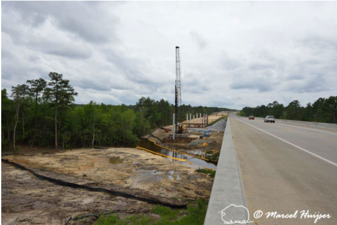
Figure 55. Erosion control at a construction site of new bridge in association with highway widening (4 lanes to 2 lanes), Hwy 331, Hwy 83 near Freeport, Florida, USA.
