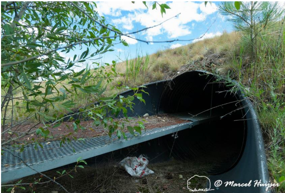
Figure 93. Shelf for small mammals in culvert originally designed for hydrology only, US Hwy 93 South, Montana, USA.
