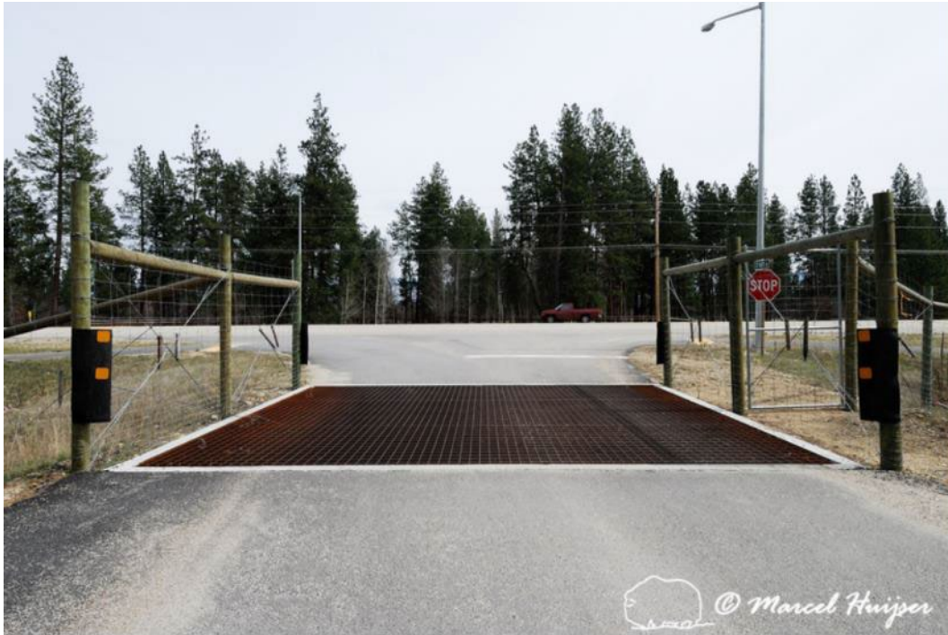
Figure 32. Wildlife guard installed at an access road to the main highway (US Hwy 93S), near Stevensville, Montana, USA. The metal barrier is easy to walk and bike over. Note that the concrete ledge can be used by wildlife to access the fenced road corridor. This concrete ledge should be made inaccessible.
