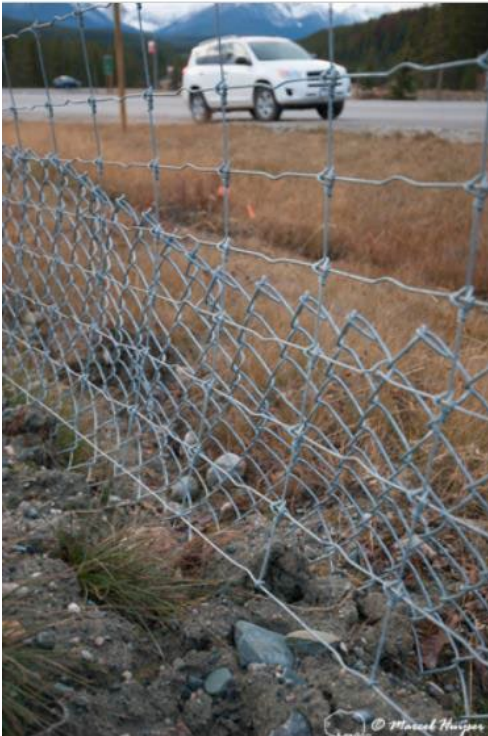
Figure 10. Wildlife fence and dig barrier (“buried fence” or “apron”), Trans-Canada Highway, Banff National Park, Alberta, Canada. The dig barrier in the soil angles (45°) towards the safe side or habitat side; it angles away from the fence and the road on the other side (Clevenger and Huijser 2011). The dig barrier keeps animals from digging under the fence. The dig barrier may consist of a 4-5 ft (1.0-1.2 m) wide galvanized chain-link fence that is attached to the bottom of the actual fence. The buried fence should extend approximately 3.5 ft (1.1 m) under the ground (Clevenger and Huijser 2011).
