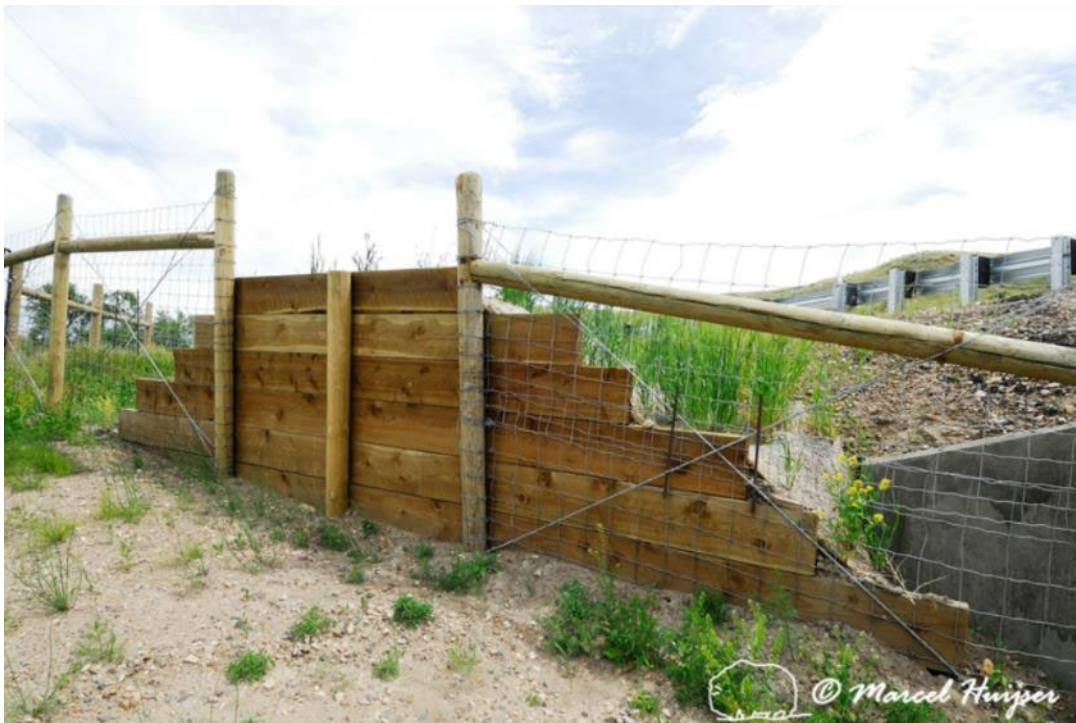
Figure 48. Wildlife fence and jump-out with a face consisting of wooden planks, near Havre, Montana, USA.
