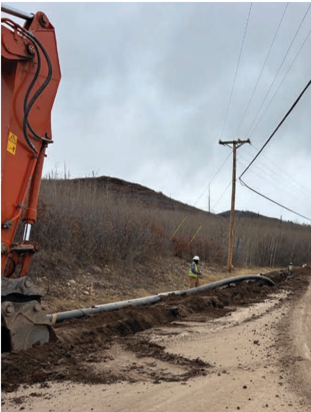
Contractor Dub-L-EE continued work on the Jemez Mountain Fire Protection Project before shutting down for the winter in mid-January.
