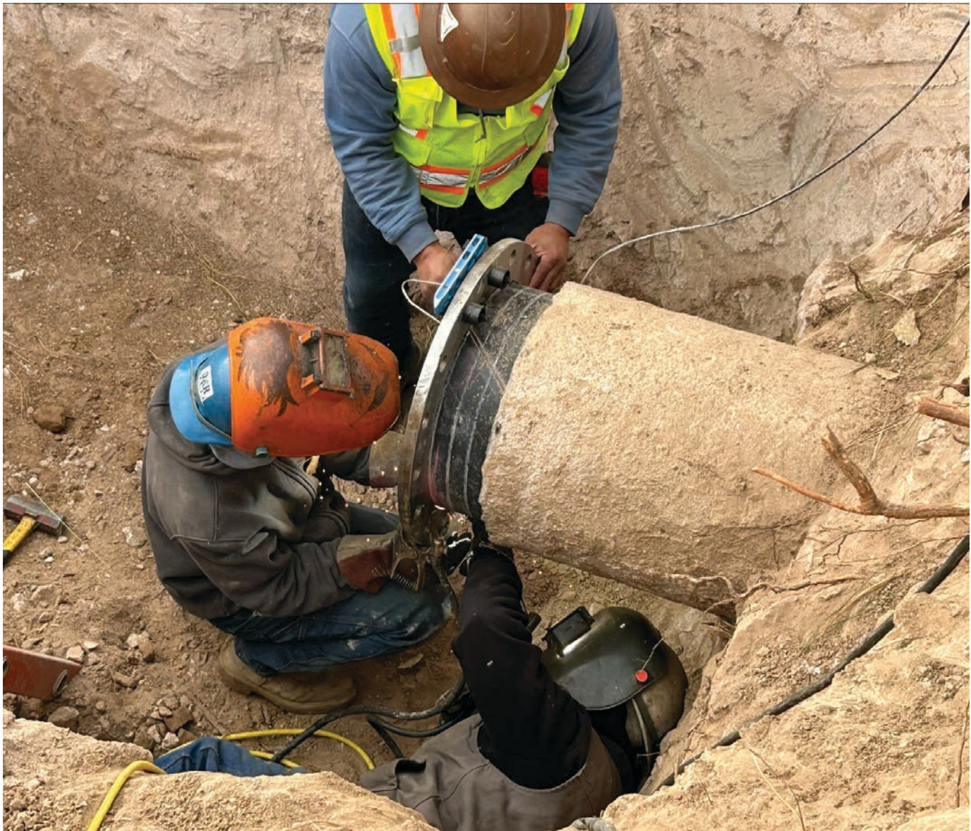
Workers from contractor File Construction and D&R Tank weld a flange to the steel core of a large water pipe.
