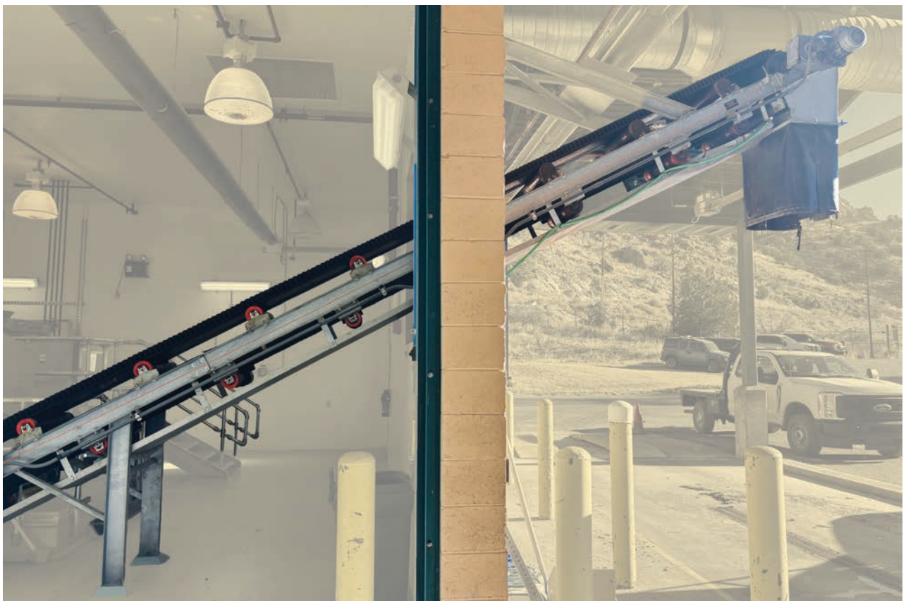
The new belt press at the Los Alamos WWTP is operational after a large replacement project.
