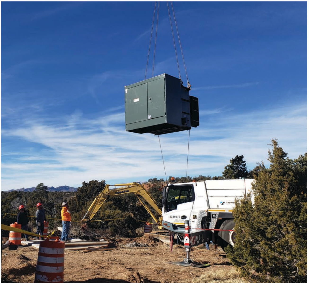
Electric Distribution staff from the DPU worked with LANL crews when a new transformer was delivered. This transformer is part of the tie line constructed between LAC and LANL in case backup power to White Rock is necessary.
